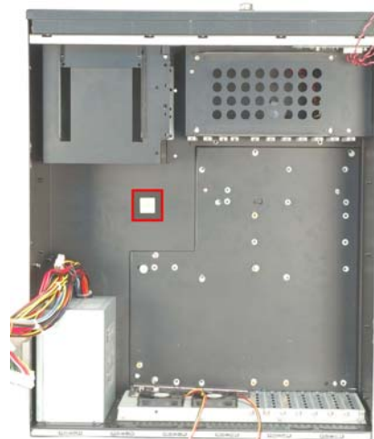
Figure 40: Plastic Pillar Stuck on the Base of the Chassis
