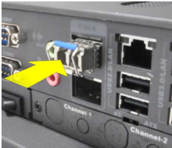
Figure 3-6: SFP Module Installation
