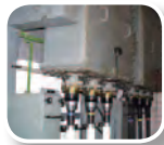
Power sensitive equipment
